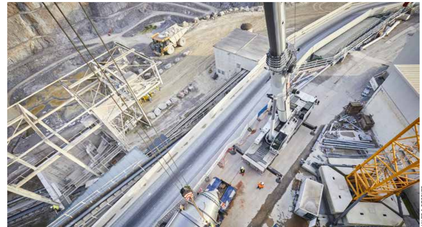
The Hahnstätten lime plant includes a new packing complex
